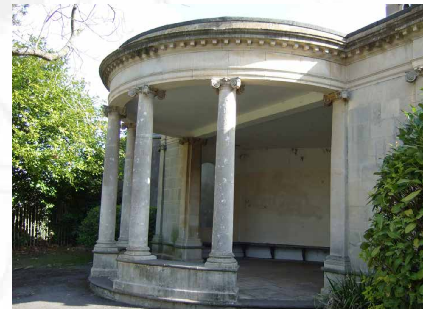
Loggia Stonework, interior and seating in need of repair. Proposal: Restore stonework and interior, provide new seating and interpretation
