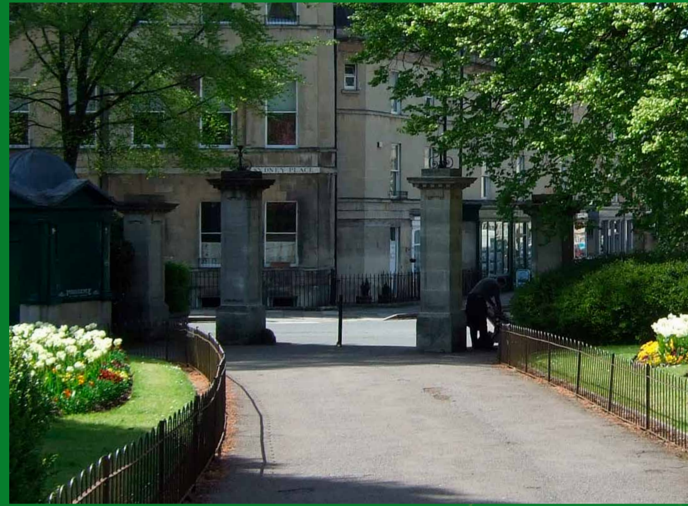
Main Entrance Historic entrance to the park, gates are missing. Proposal: Restore framework including fittings, replace gate
