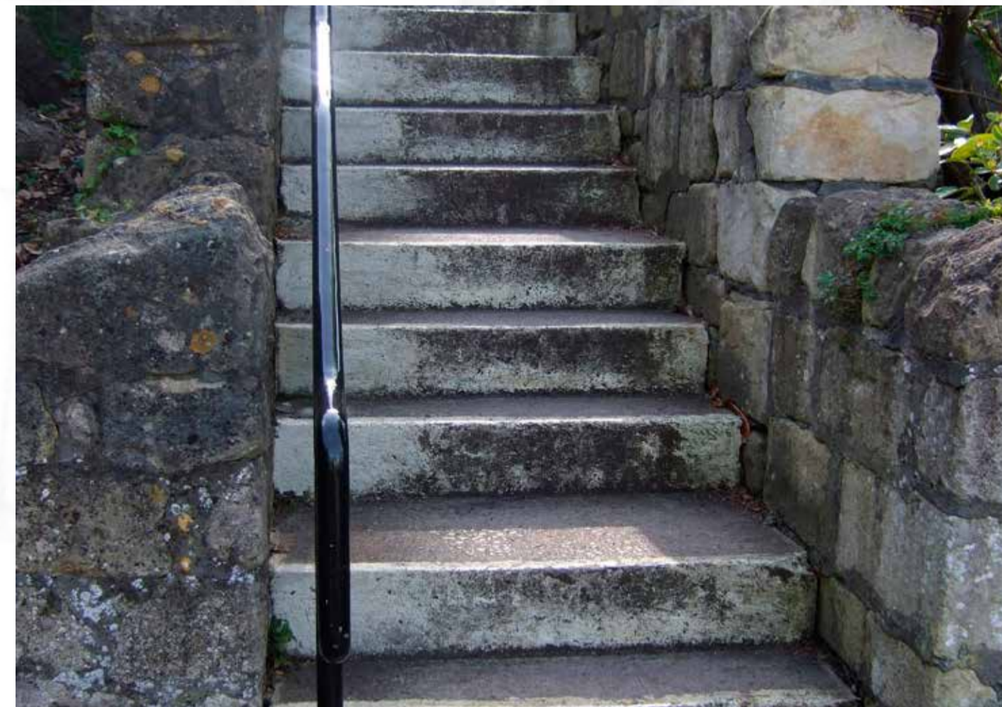
Stepped entrance from Sydney Road Access is very steep and narrow. Proposal: Widen entrance
