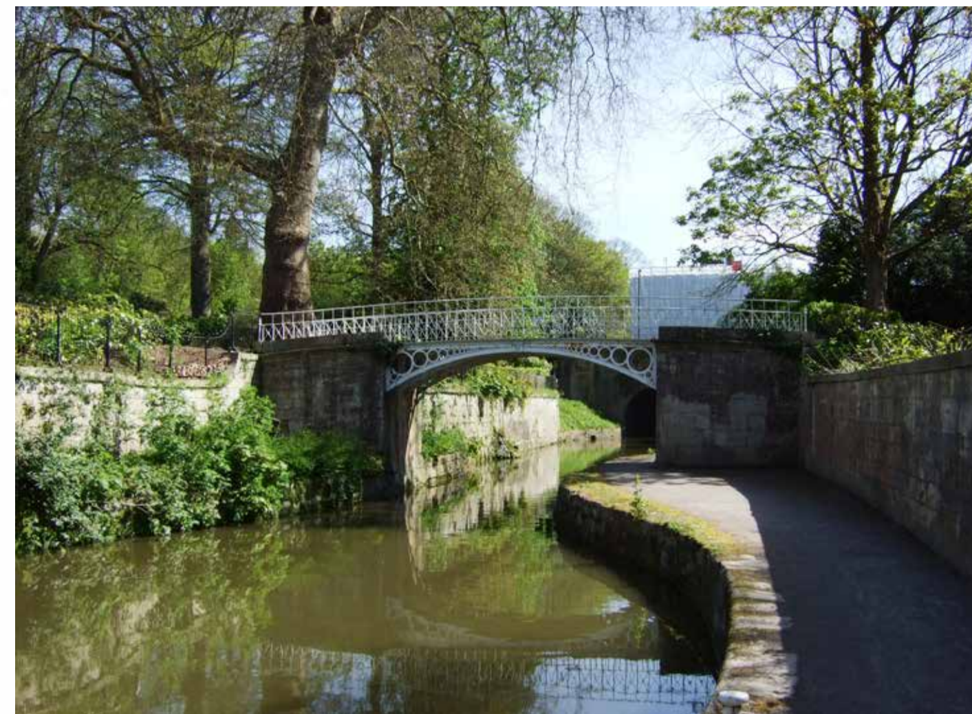
Canal Bridges (G & H on Plan) Ornate metal railings to both canal bridges in need of repair. Proposal: Restore and repaint
