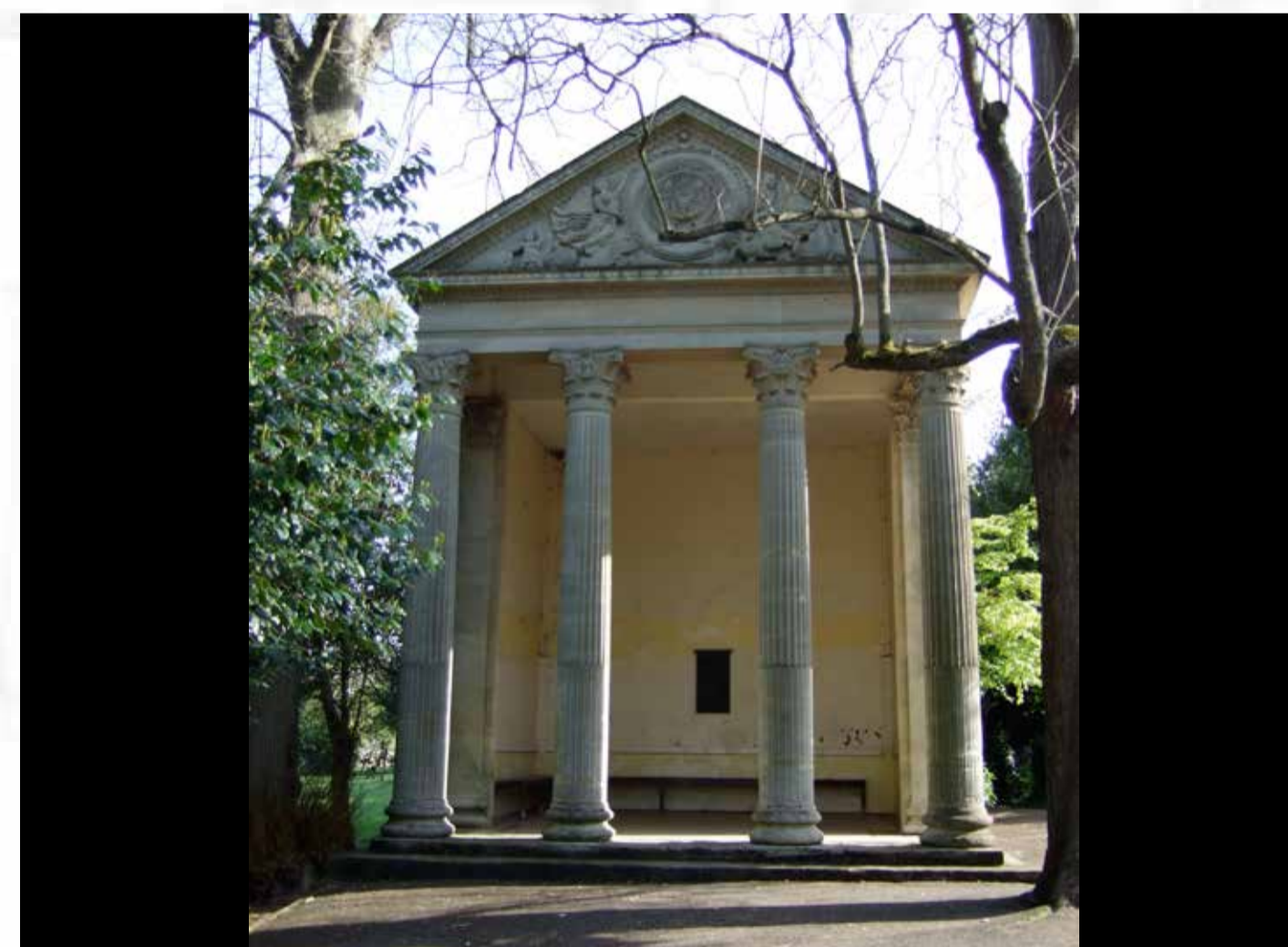
Minerva's temple Stonework, interior and seating in need of repair. Proposal: Restore stonework and interior, provide new seating and interpretation
